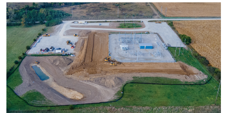
The expanded footprint of MPW West Substation is the starting point for Line 106.
