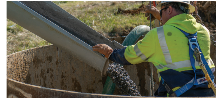
Hahn Ready Mix pours the concrete for one of the steel pole locations.
