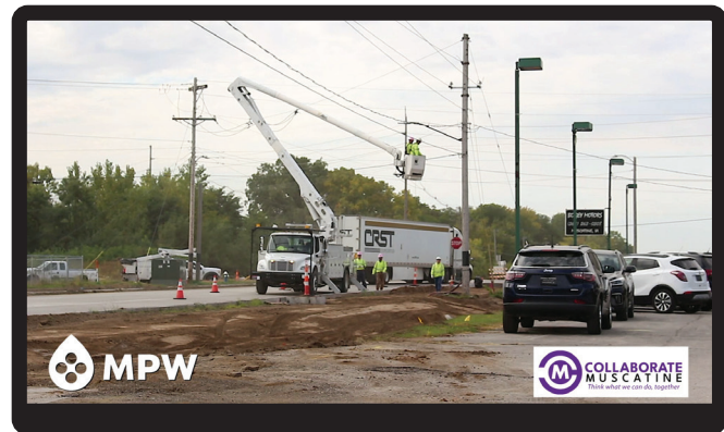
On Grandview, all three utilities enhanced reliability; with water main and valve replacements, and undergrounding on overhead electric and communications lines.
