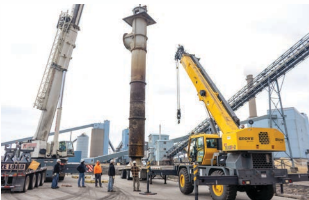
In November 2025, a Circulating Water Pump is lifted for refurbishment, part of MPW's commitment to reliable, efficient power for years to come.
