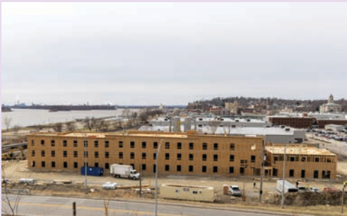
Progress continues at Lumber Lofts, where new housing is taking shape with MPW-supported electric, water, and communications infrastructure.
