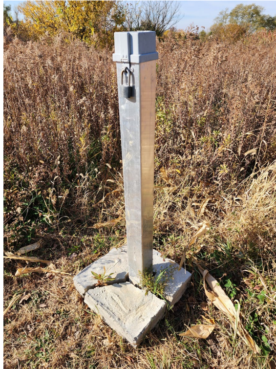
Photo 1 Broken concrete pad at monitoring well MW-26.
