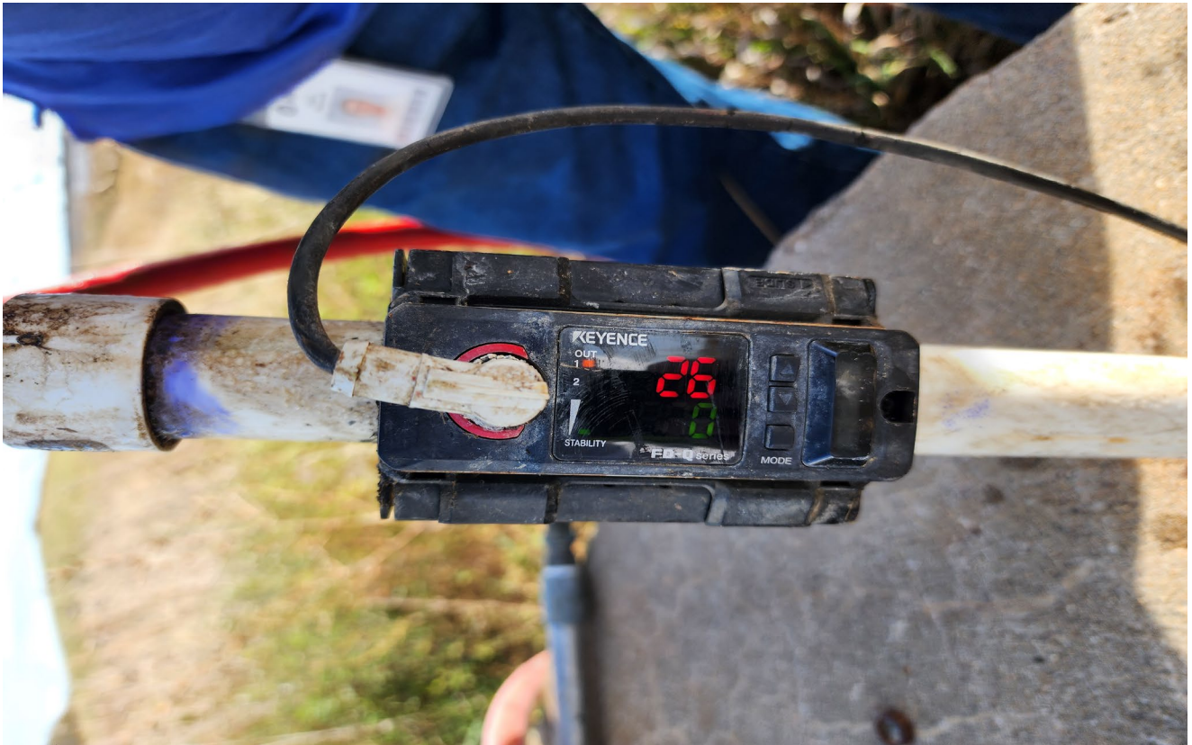
Photo 4 Leachate discharge totalizing flowmeter reading 260,000 gallons.
