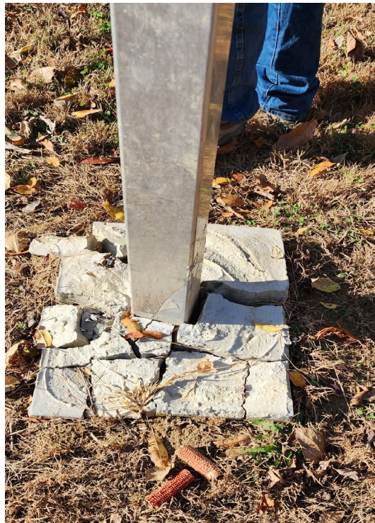
Photo 2 Broken concrete pad at monitoring well MW-27.
