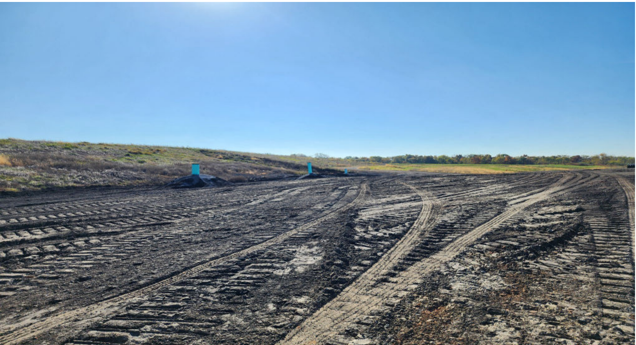
Photo 4 Active filling area with stormwater management structures to the left. Looking south.
