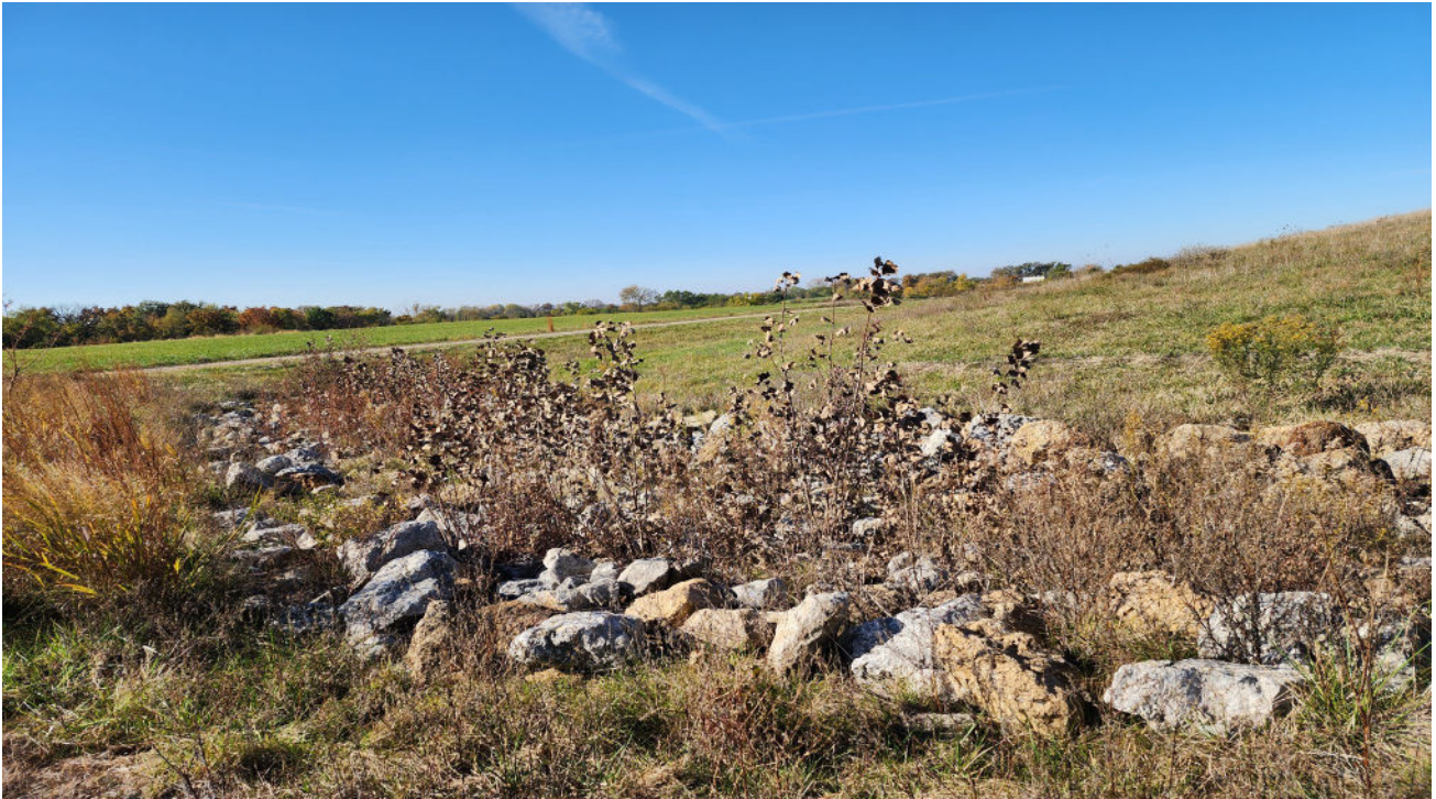
Photo 3 Rip-rap drainage collection area at southeast corner of landfill with vegetation growth. Looking southwest.
